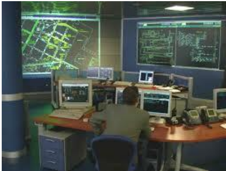
Figure 10 - Energy Control Room of IRN
