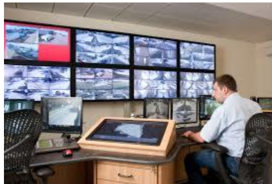
Figure 2 - A control Room
