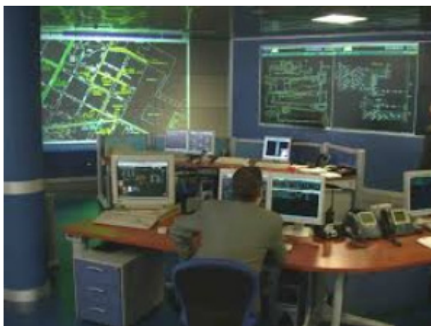
Figure 4. The Energy Control Room of IRN
